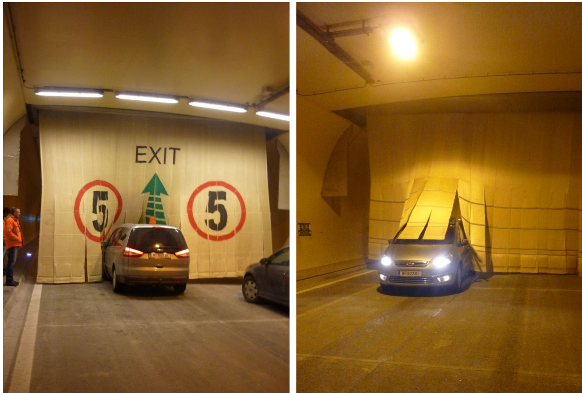
Figure 4 Flexible curtain that is lowered in case of fire in the Roppener tunnel, Austria
